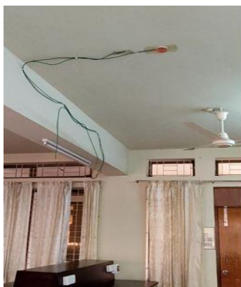
Fig.3 Heat flux sensors in the air-conditioned room.
