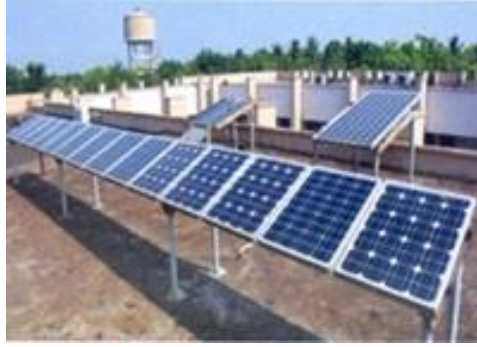
Figure 5: Solar Panel, KUET
